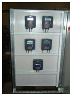
TDS Bleed control board
